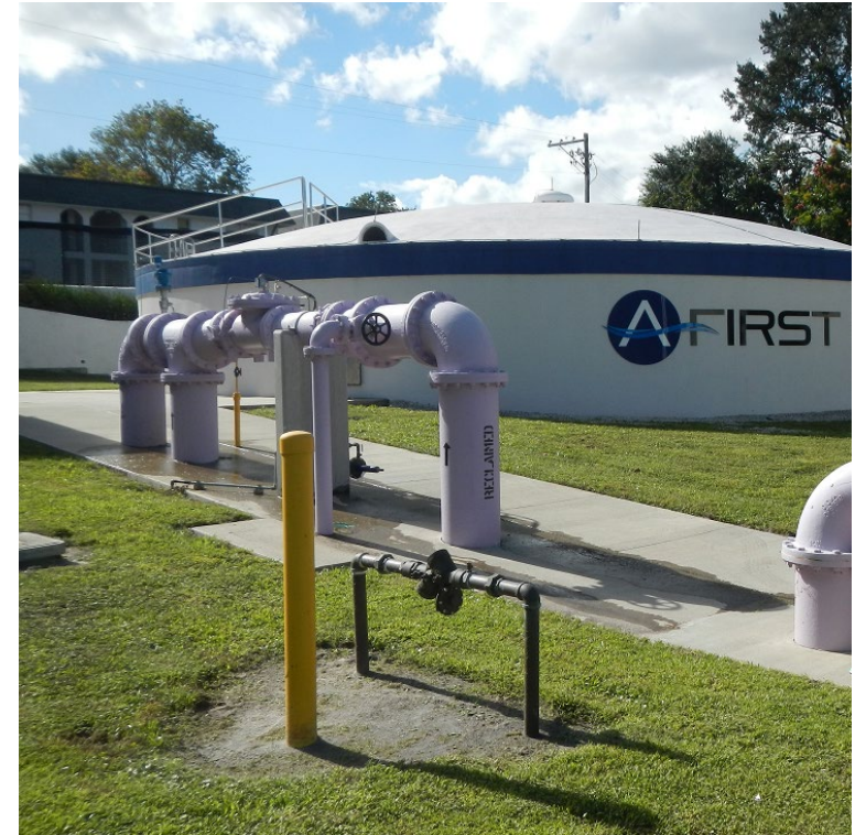
Altamonte Springs-FDOT Integrated Reuse and Stormwater Treatment (A-FIRST) capture and treats stormwater from a nearby highway to be used for irrigation.
