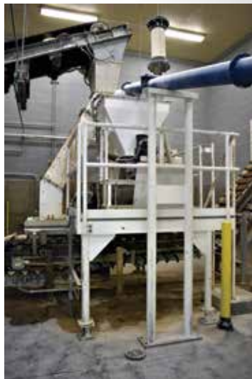
2018 Nutrients Permitting Workshop, Tussing Road Water Reclamation Facility, Pickerington, OH Katie Foreman, Association of Clean Water Administrators
