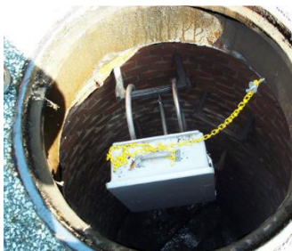
Flow meter with communication technology.
